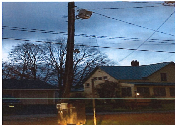
Abandoned light pole and electric meter
