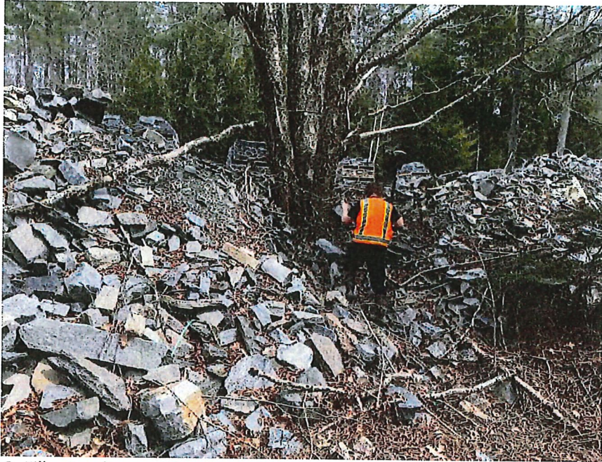
Photo 3: Fill extending past large tree. Location of tree indicates previous break in slope
